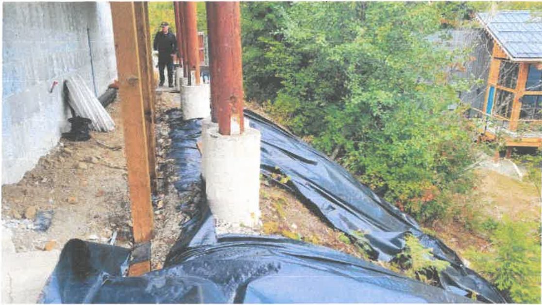
Looking west along north wall, demolition work continues and protecting slope with plastic.
